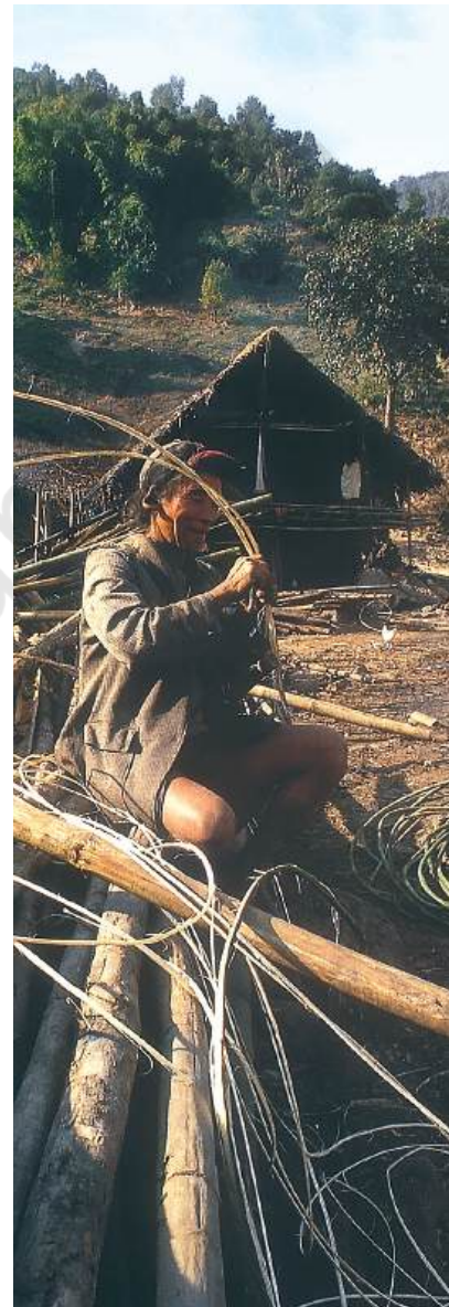
Fig. 5 – A log house being built in a village of the Nyishi tribes of Arunachal Pradesh.
